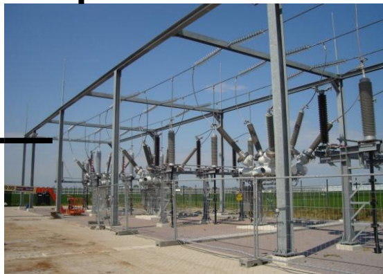
Power station (250 MW)
